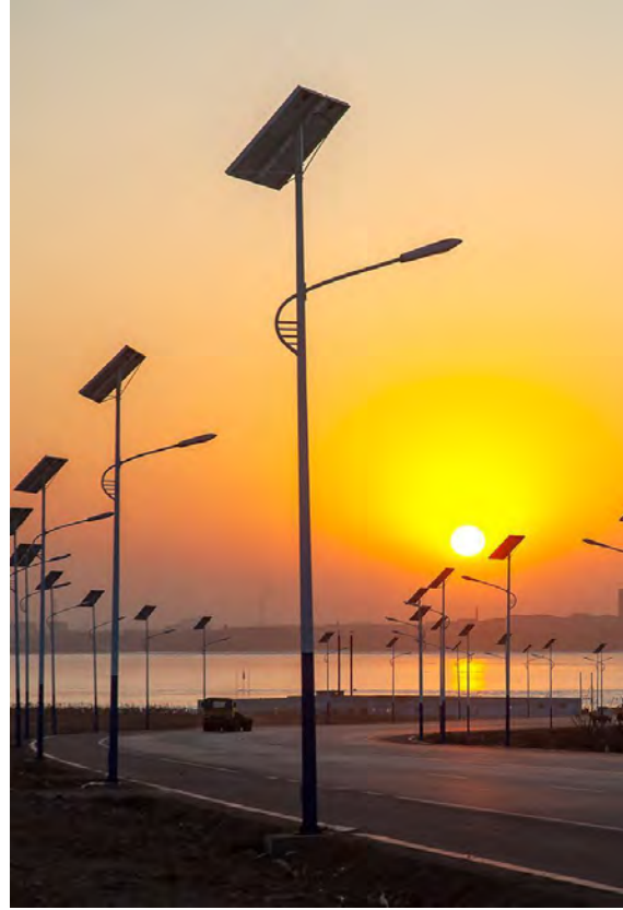
Smart Solar Street Light Control
